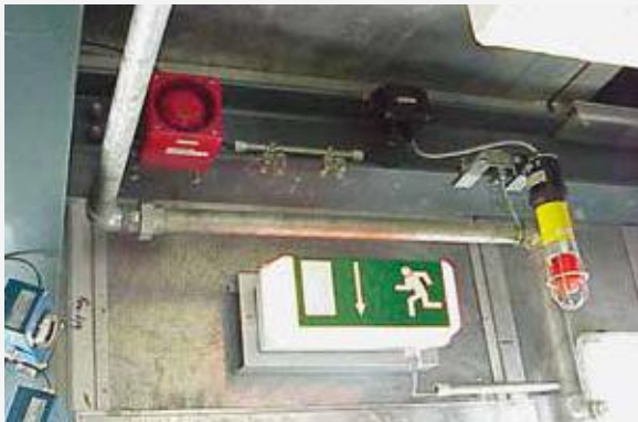
Gas detection with visual and acoustic alarms: 🔊 sounder DS 10 ATEX and 🚨 flashing light CWB-ATEX.
